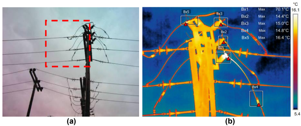
Fig. 4. (a) The visual photo of a disconnector and (b) the thermal photo of the same disconnector reveals the most common problem, a fault with the connection at the top of the bushing
