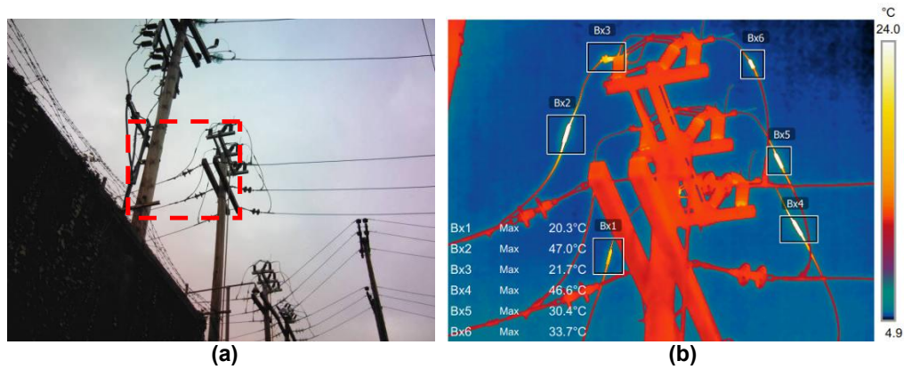
Fig. 7. (a) A visual image of a 3-phase disconnector and (b) the thermal photo shows problems faults in the input of A-phase and in the output of C-phase
