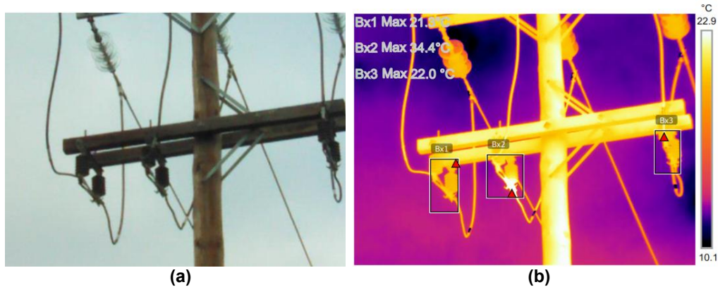
Fig. 5. a) The visual photo of a 3-phase knife switch shows and b) the thermal photo which reveals a fault with priority 3
