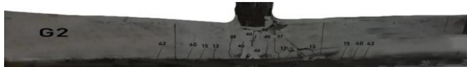
a) Cracking Patterns for Beam (G2) [EXP]
